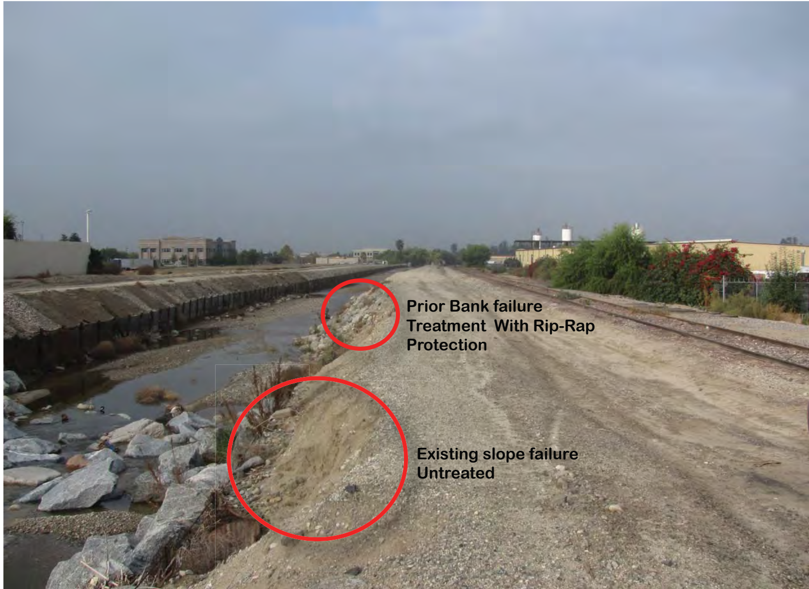
Mission Zanja Channel Bank Failure
