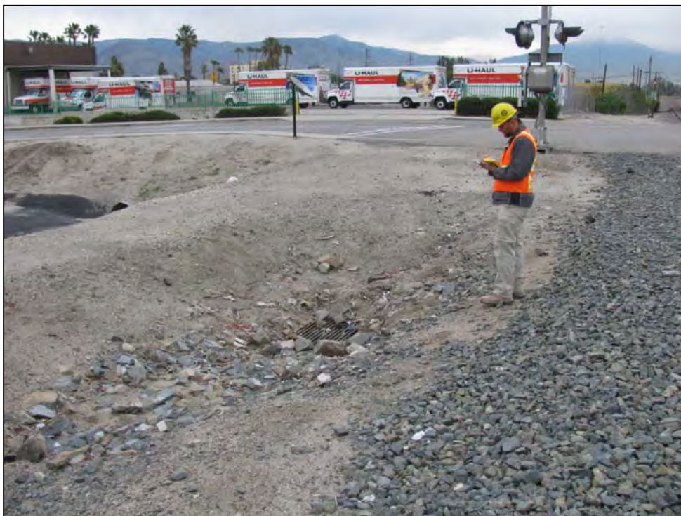
Photograph 10. Stormwater from adjacent urban areas channels into the railroad ROW and is transported through a series of culverts into larger drainages.
