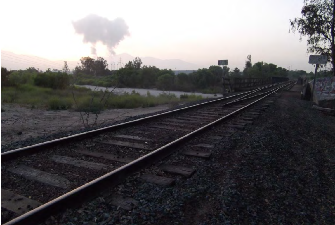
Photo 3. Standing on north side of SAR as rail road approaches abutment looking southeast.
