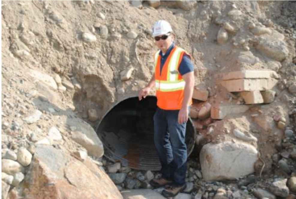
MP 5.2, 24-inch RCP (no. 4)
