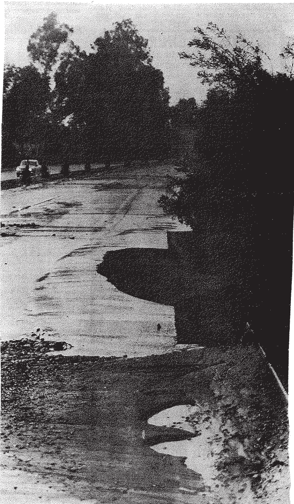
BOULEVARD COLLAPSED —Severe flooding undermined and collapsed this portion of Redlands boulevard in the eastbound lanes between New York and Tennessee streets. Motorists who were able to travel the road after nearly two feet of water drained off found they had to dodge rocks and other debris, as well as thick, slick deposits of mud. (Photo by Dick Wiley)
