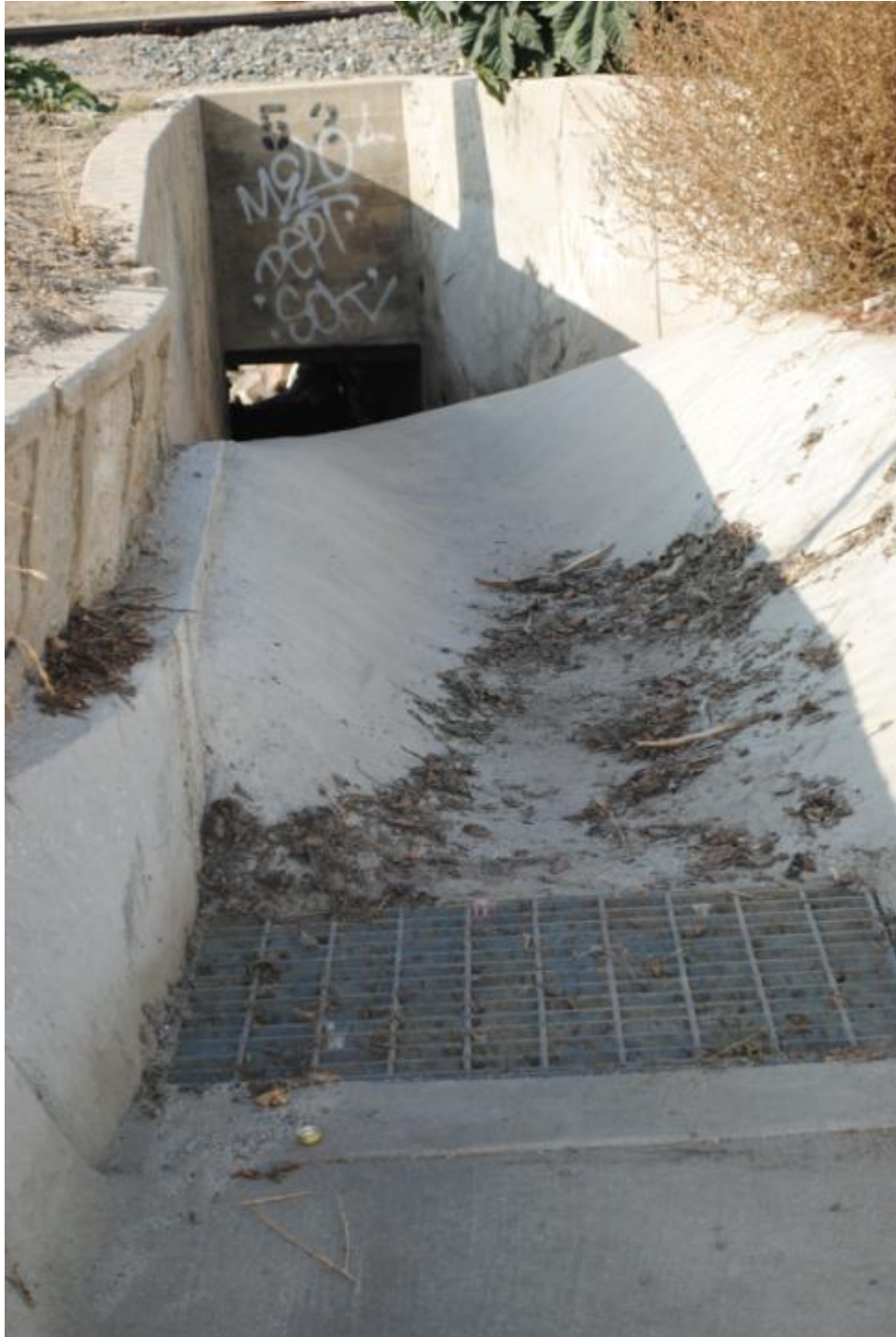
MP 5.2, 24-inch RCP (no. 1)
