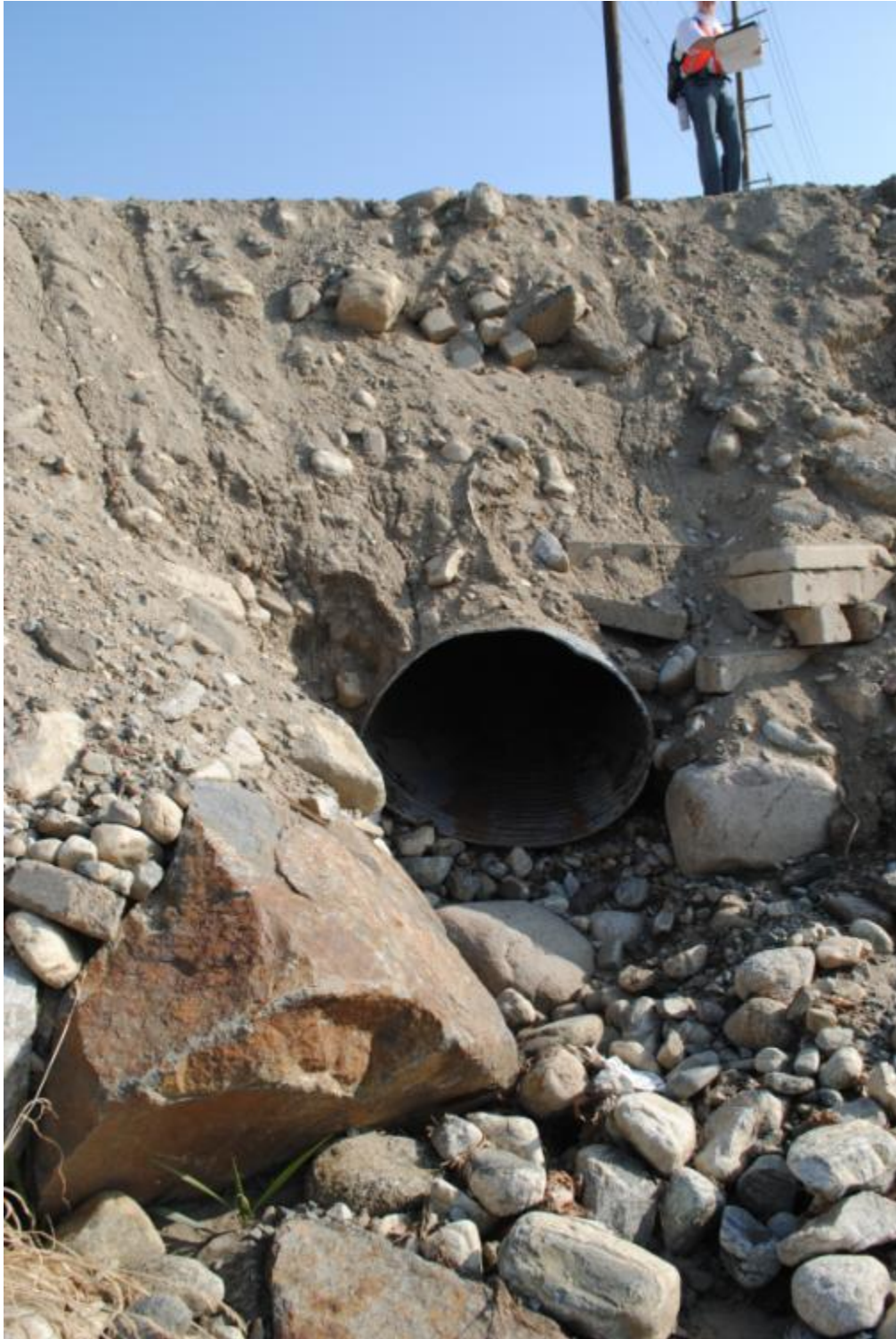
MP 5.2, 24-inch RCP (no. 3)
