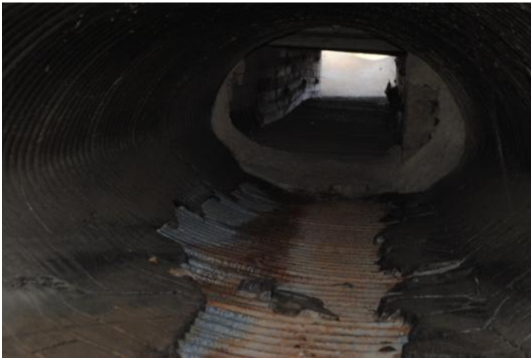
MP 5.2, 24-inch RCP (no. 5)
