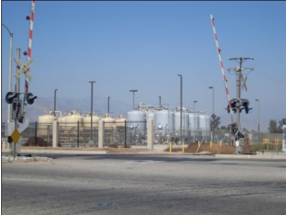
Photo 3: Raub GAC treatment facility located at Waterman Avenue (Map Code AD). View is toward the northeast.
