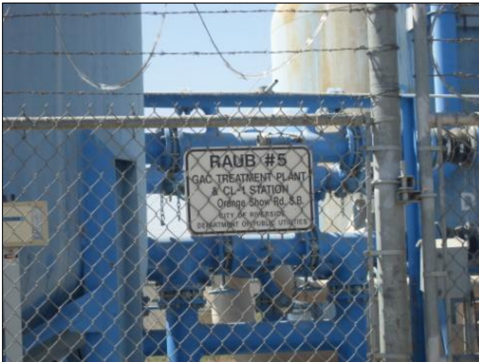
Photo 4: Raub GAC treatment facility located at Waterman Avenue (Map Code AD). View is toward the northwest.
