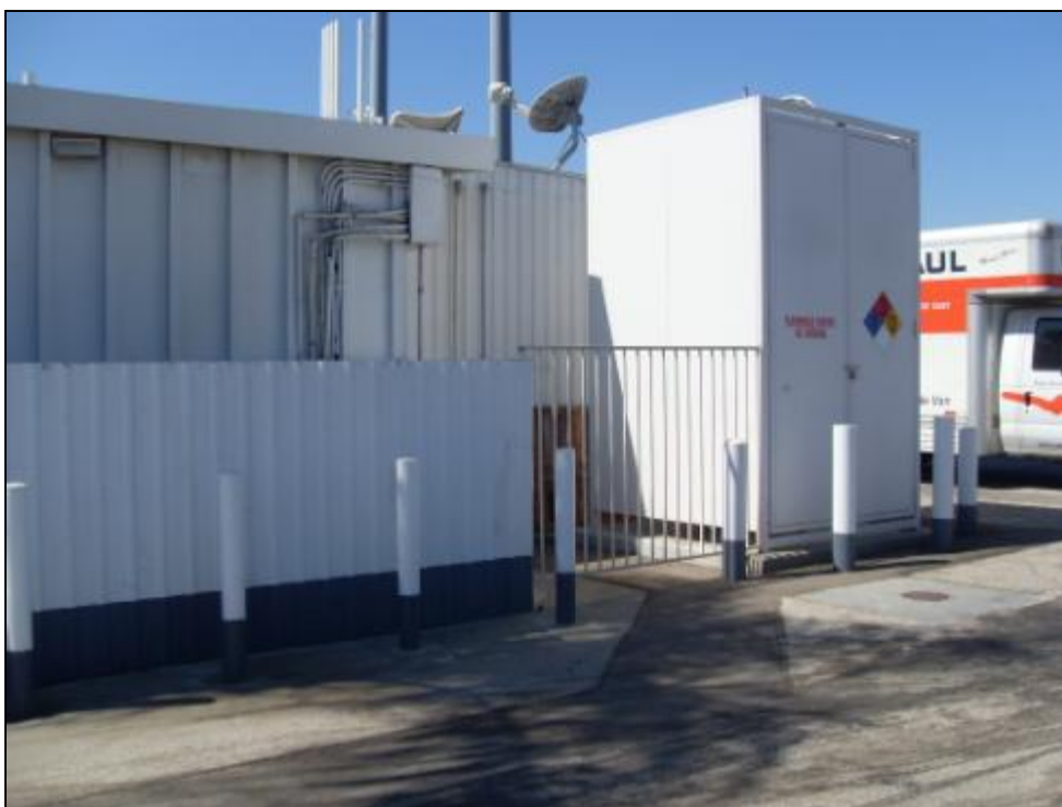
Photo 8: Remediation system and curb cuttings located at Shell Station. View is toward the southwest.
