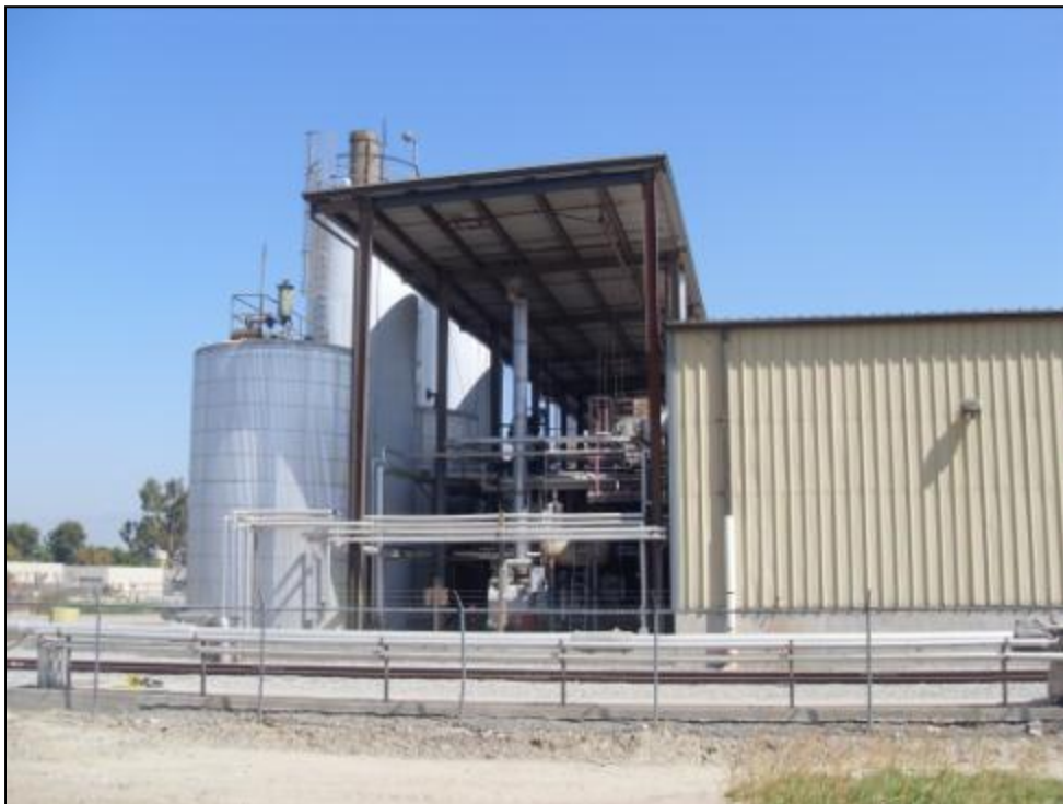
Photo 6: Aboveground storage tanks (ASTs) and piping located at the White Flyer facility (Map Code D). View is toward the northwest.
