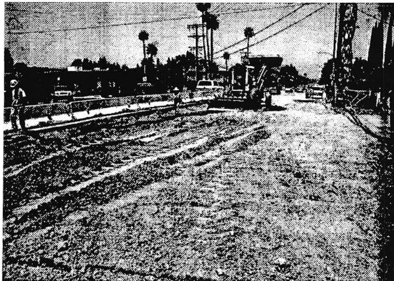
SOJV subcontractor Romero started rough grading, Phase 3 of intersection work at De Soto Avenue.
