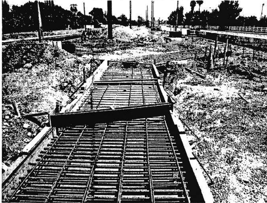
SOJV subcontractor Rainbow continuing installation of storm drain culvert near Mason Avenue.
