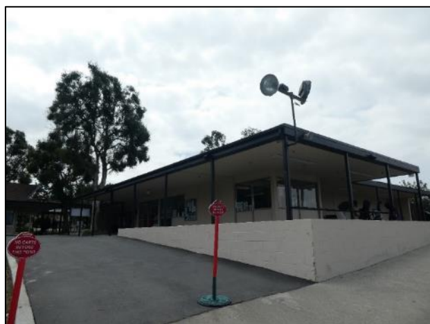
Figure 10. View of the north elevation of the western section, view facing southeast. Note the projecting rectangular portion of the walkway, the concrete block retaining wall and asphalt walkway. Source: GPA Consulting 2019.
