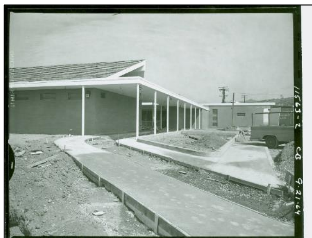
Figure 18. Photo showing the south elevation of the western section and the projecting rectangular mass on the south side of the eastern section, view facing east. Source: Calisphere, September 21, 1964.
