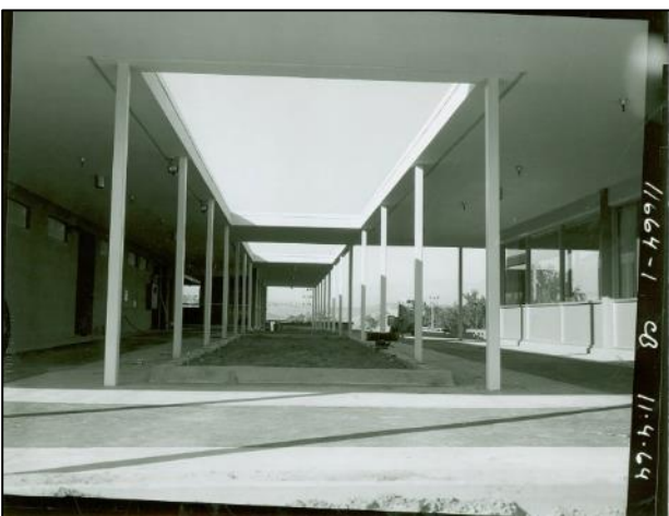
Figure 19. Photo showing the rectangular gardens and cut-out roof motif while under construction, view facing north. Source: Calisphere, November 4, 1964.
