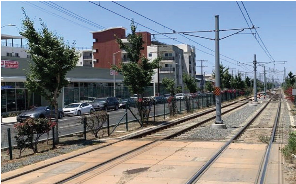
Figure 1-5. Example of Overhead Catenary System
