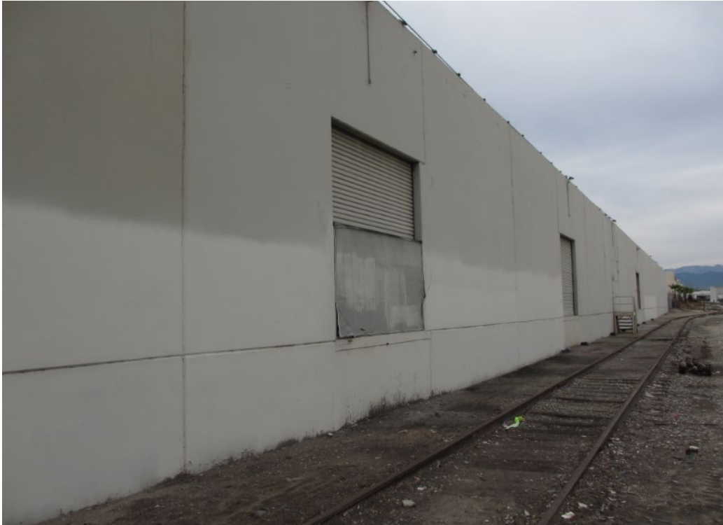
Figure 6-15. Goodyear Tire and Rubber Company Warehouse constructed 1952 and Existing Rail Alignment Facing Washington Boulevard (2353 Garfield Avenue) View East
