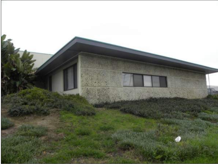
Photograph 2. View of north elevation of office portion of building, camera facing south, 12/18/2019, DSCN0253
