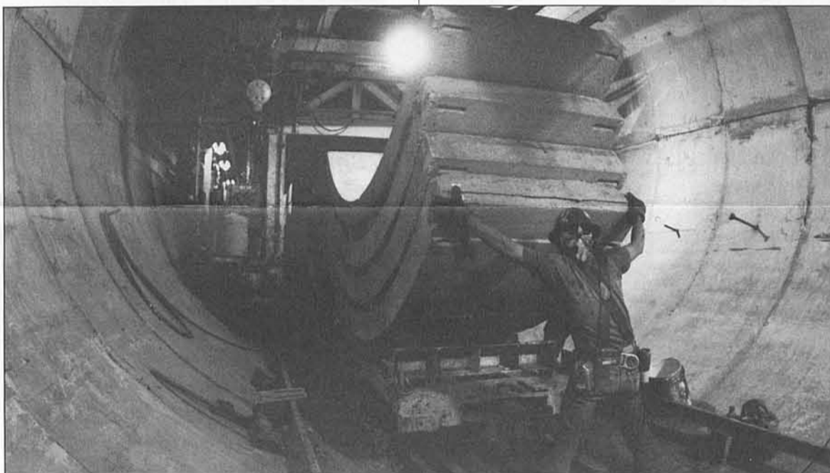
Cast of thousands — A worker delivers some of the thousands of pre-cast concrete segments installed during heavy construction in 1988. The Red Line’s tunnels are actually double-thick — built with two layers of concrete.
