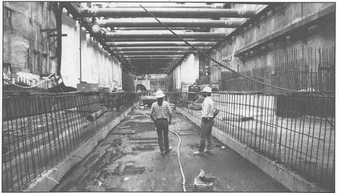
Underground — Workers walk through the subway station construction site below the intersection of Wilshire Boulevard and Vermont Avenue. During construction, vehicles continue to pass above on planked streets.
