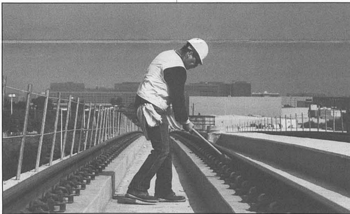
Clipping along — A construction worker on the Metro Green Line's El Segundo aerial bridge fastens rail strips to concrete ties with thick steel clips.
