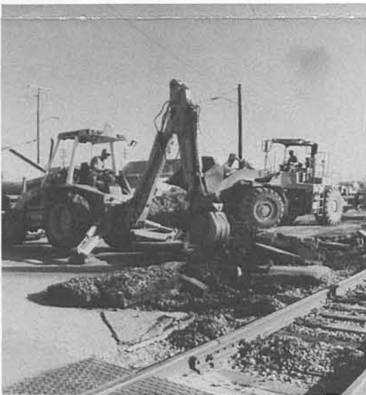
Lancaster Station where crews worked around the clock to get track ready for Metrolink trains.
