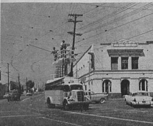
ELECTRICAL —Emergency Tower Crew rebuilding curve in trolley wire at Jefferson and San Pedro. Harold Jones, left, and Richard Jellison are atop the tower truck.
