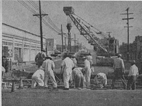
WAY & STRUCTURES —Special Work Gang under Foreman Carl Heffington removes a crossing at Vernon and Hoover Sts. and replaces it with 116-lb. rail.
