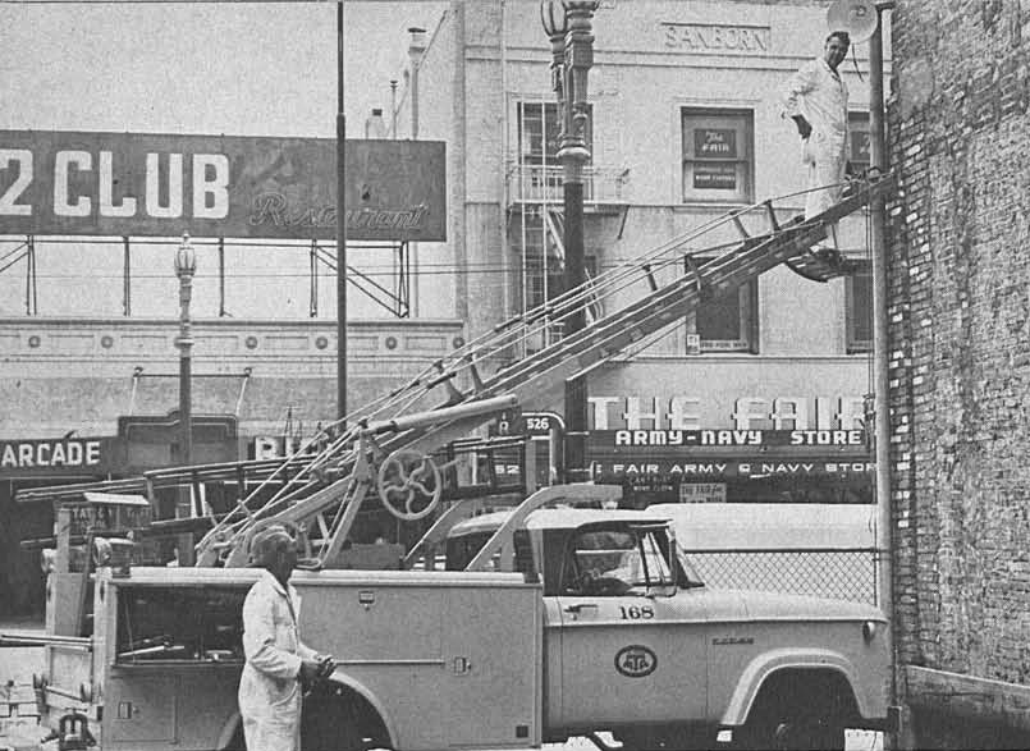
TAKING DOWN OLD YARD LIGHTS on lots at Terminal 16 are Electricians T. W. ("Tommy") Thompson (on ladder) and Jim Thagard. Brighter and better floodlights will be installed in the yard.
