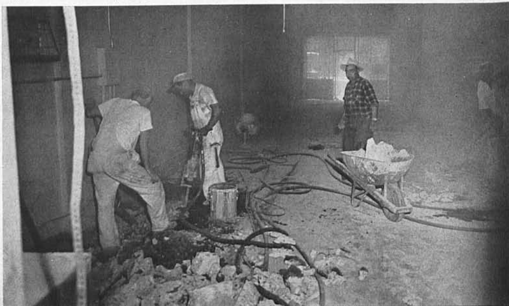
DUSTY JOB —Work of renovating the buildings at Terminal 16 for use as station is under way. These employees of the Property Maintenance Department are tearing up the floor in order to lay additional plumbing. You may not recognize their faces for dust, but they include, from left, Leadman Bill Corwin, and Mechanics Sam Galatioto, Jose Aguirre (with wheelbarrow), Salvador Burgos, and Ynz Nunez, Concessions, restrooms and Information Counter will be in here.
