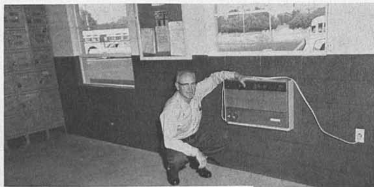
ABOVE —Operator E. L. Worsham, tops in Riverside seniority (5-29-26) shows off combination heater-air conditioner. AT LEFT , a glimpse of the new lockers. AT RIGHT —Operator H. E. Anunson cleans up in the bright new washroom.
