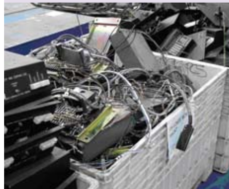
Incompatible PA systems and wiring were removed from all 69 Blue Line trains.
