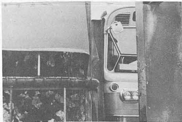
A fine steady spray of water keeps the dust from 5937 from polluting the surrounding area. As the debris is sucked from the bus it all goes into the wire-like cage at left.
