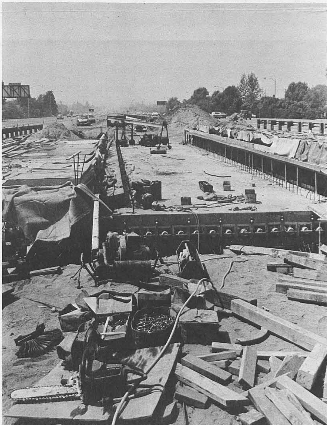
BUSWAY CONSTRUCTION MOVES RIGHT ALONG—Concrete barrier walls (top photo) constructed to separate the Busway lanes from the Southern Pacific Railroad tracks rapidly take shape. Busway lanes 17 feet wide will parallel the barriers with a line of brightly colored rubber pylons on the outside of the lanes. A 20-foot shoulder between the pylons and the freeway's number one lane will be used as an emergency parking area for Busway buses and freeway vehicles. Overpasses, such as the one at San Fabiel Boulevard (bottom photo) are being modified for the Busway. Some overpasses had to be reinforced while others needed to be widened.
