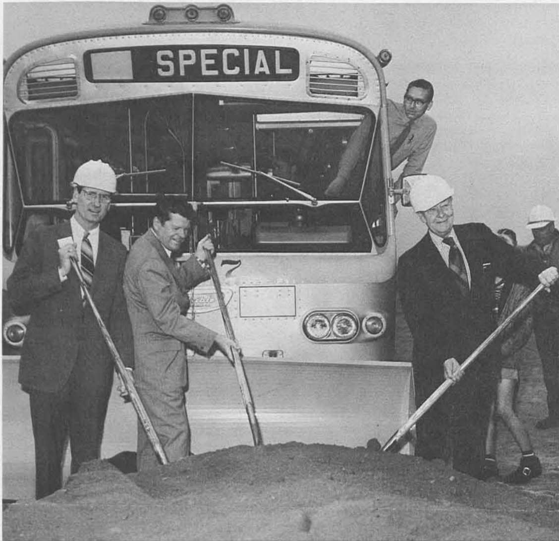
Frank J. Walton, California secretary of business and transportation, County Board of Supervisors Chairman Warren M. Dorn and RTD President Norman Topping, take the first shovels full of dirt to commemorate the beginning of construction on RTD's El Monte-Los Angeles Busway.
