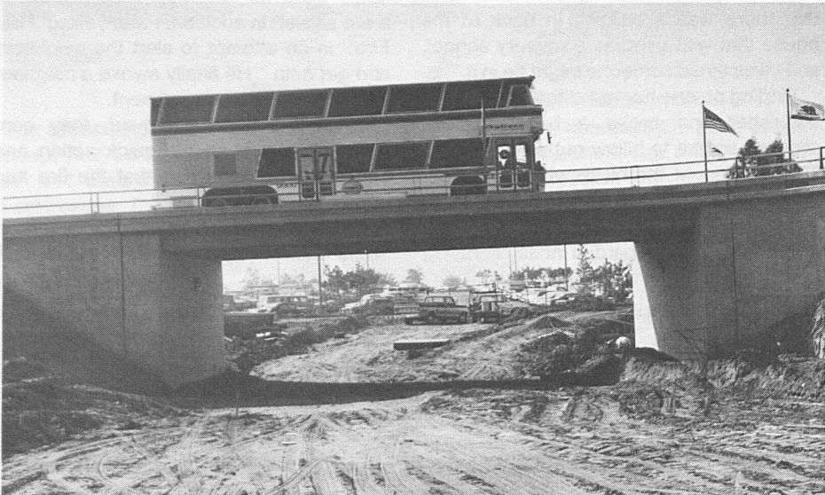
STARTING FROM SCRATCH —Construction is now underway of the east parking lot at the El Monte terminal. When completed, the new parking lot will provide an additional 700 patron parking spaces, and will also have an access road leading under the bridge to the west parking lot. The south access road, currently being used by both buses and cars, will be reserved for buses and will also provide direct access to the maintenance facilities at the adjacent Division 9. The bus in the picture is RTD's double decker, pulling into the El Monte Terminal after a trip on the Busway.
