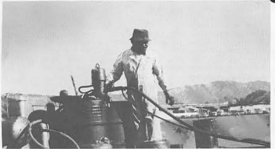
Walter Brown, a laborer "A", keeps a watchful eye on the asphalt process from a flat bed compressor truck.
