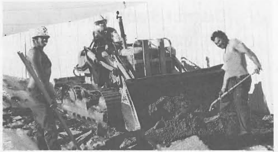
Ron Foss, (left), Henry Crossland, (center), and Jose Gomez, (right), all maintainers "A's", work as a team to cut a trench for a water culvert in the Division 15 yard.
