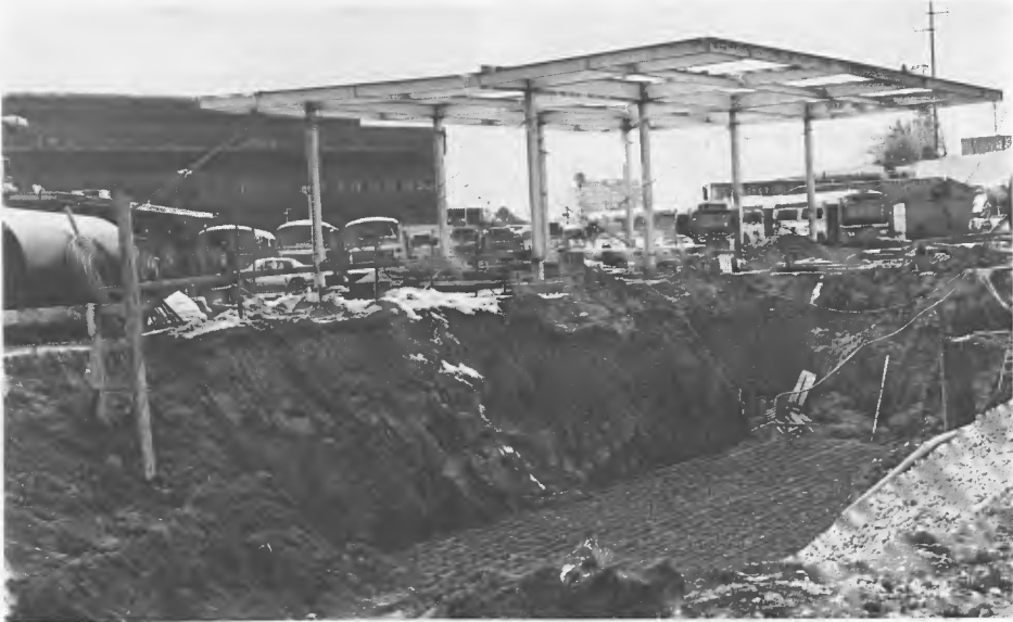
This is a close up of the excavation for the fuel tank storage 'farm' which will eventually house 20,000- and 10,000 gallon fuel tanks. The grid at bottom of the pit is the reinforcing steel for the concrete slab which will support the tanks. The steel structure in the background will be the bus washer facility.
