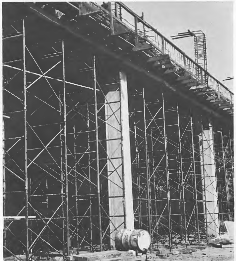
This is a close up of one of the ten bus bays. Each bay is 34 feet wide and will hold two buses. There will also be one double bay for tire repair.
