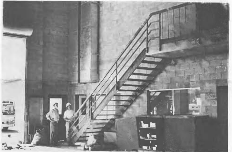
This is the interior of the new garage for bus maintenance and repair. The stairway leads to the mezzanine level which will house the lunch room, classroom and locker rooms. The office and spare parts will be on the ground floor.
