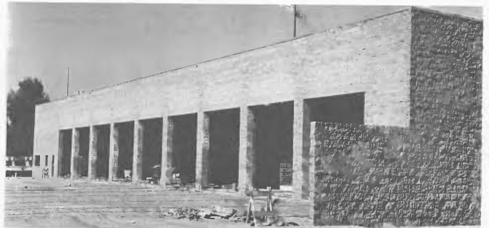
The new structure is constructed of split face concrete masonry units with tapered steel girders to support the roof.
