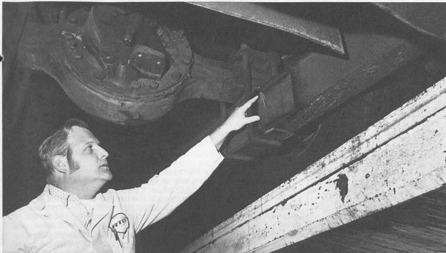
FRAMED — Equipment Maintenance Supervisor Gary Eller indicates the spot on the main frame, behind the rear axle, where cracks have developed in more than 55 per cent of
