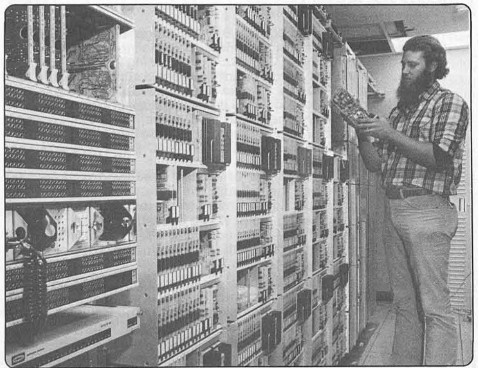
COMPUTERS — Art King, from Telecommunications, double checks one of the components in the new TRANSMIS system.
