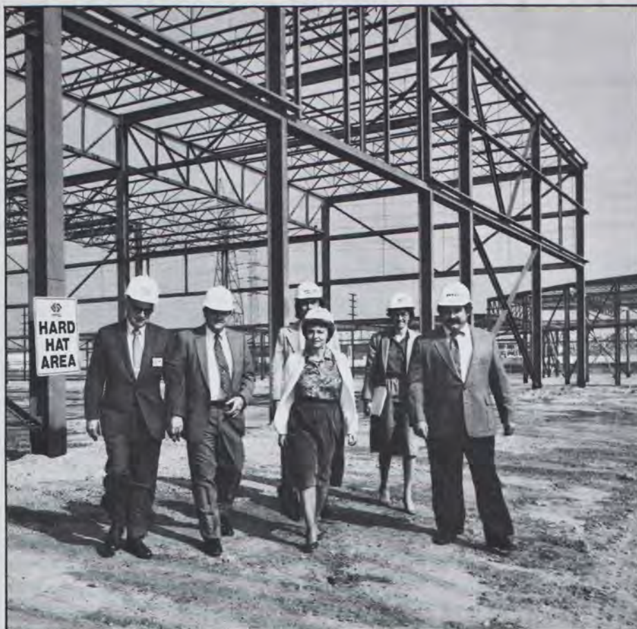
RTD Operations, Maintenance, and Bus Facilities personnel escort the new LACTC Chairwoman Jacki Bacharach through the construction site of the new Central Maintenance Facility.
