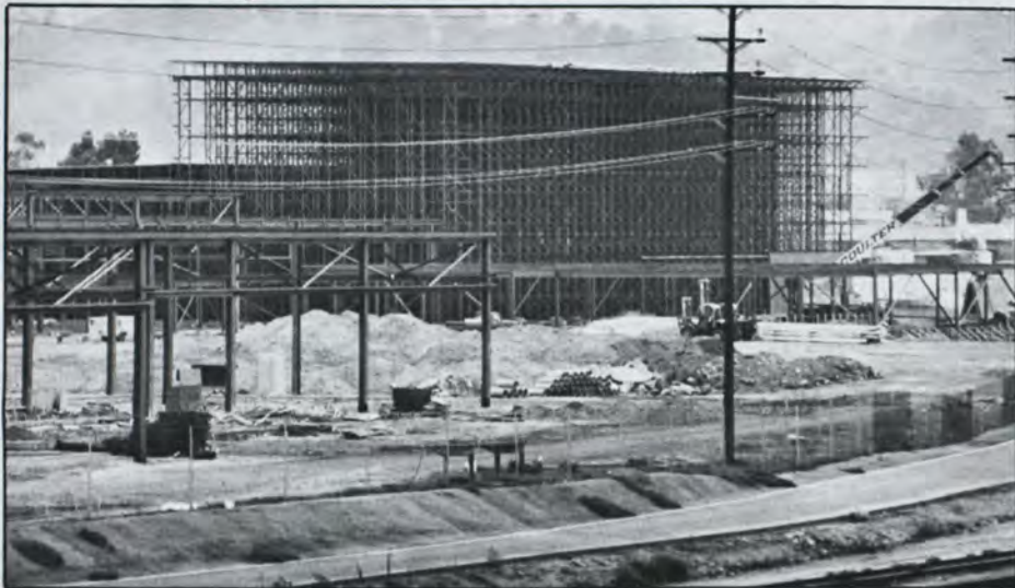
The new Central Maintenance Facility—a grid of iron girders. We'll take another look at their progress this summer.
