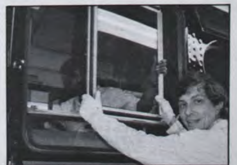
Jose Barron and Bob Pfile install a new sliding side window on a refurbished bus.
