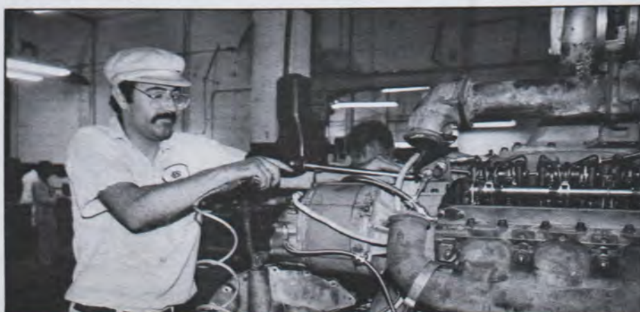
Ricardo Sylva assists in rebuilding an RTS II engine in South Park's Engine Shop.
