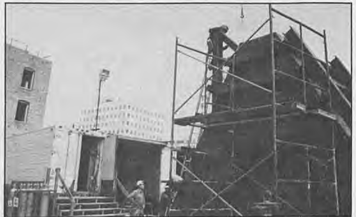
Metro Rail construction site at 7th and Bonnie Brae Streets. Workers complete welding on an earth hopper which will load the muck encountered from excavation work.
