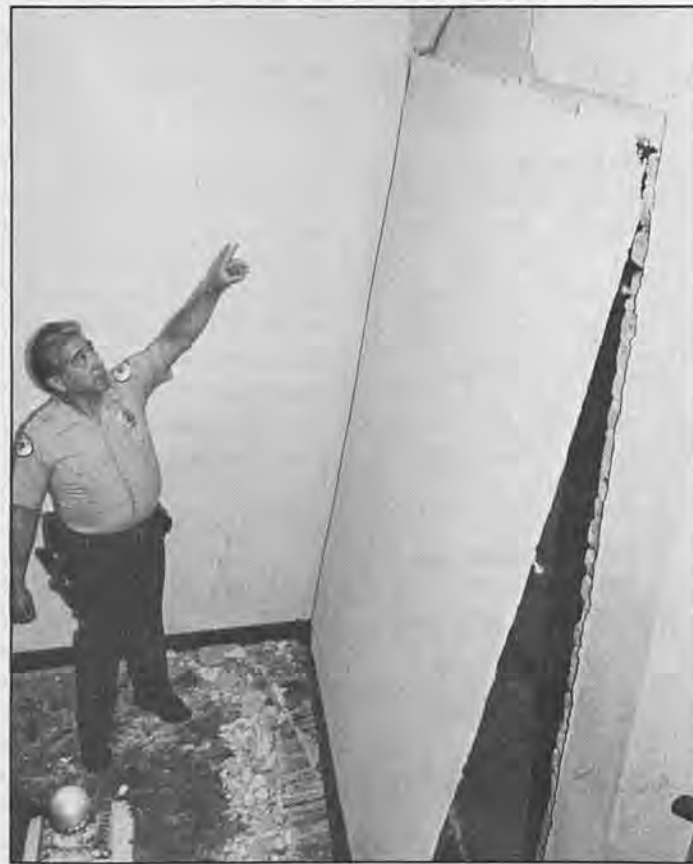
Security Guard Anastacio Puente points out damage in the stairwell of the 411 Main Street Building.
