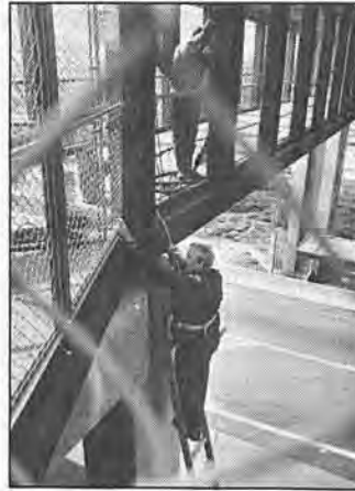
RTD Engineer John Joyce, on a ladder 30 feet from the street level, examines the underside of the University Bus Station bridge to ensure that it is safe for alighting RTD passengers.
