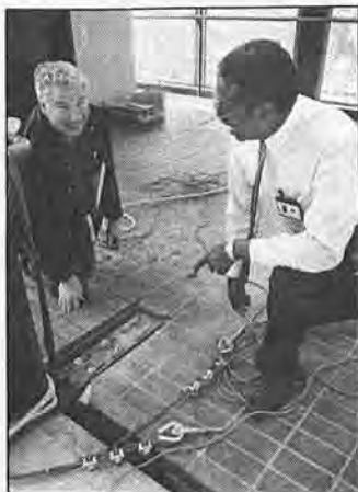
RTD Bus Facilities Engineers John Joyce (left) and Elmo Douglass (right) inspect the repair work done at the Cal State University Bus Station.
