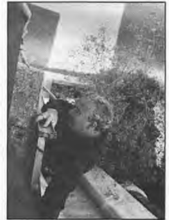
RTD Engineer John Joyce's view from the bridge includes an inspection of all sides and surfaces of the structure.
