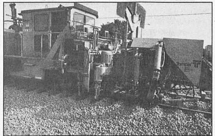
A ballast tamper and track leveler machine on the right-of-way along Long Beach Avenue lifts the rail previously laid and levels rail using a laser device while simultaneously re-tamping the ballast underneath the rail to ensure a firm foundation and to prevent settling.
