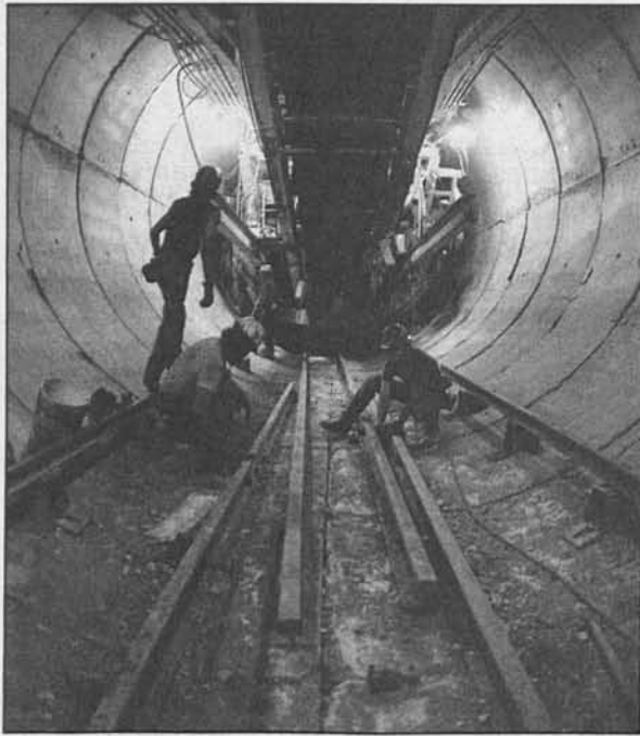
Tunnel workers lay the concrete liners as the tunneling machine digs ahead of them. The muck unearthed is transported overhead on a conveyer belt. (Photo by Jost/Alfvin Photography)
