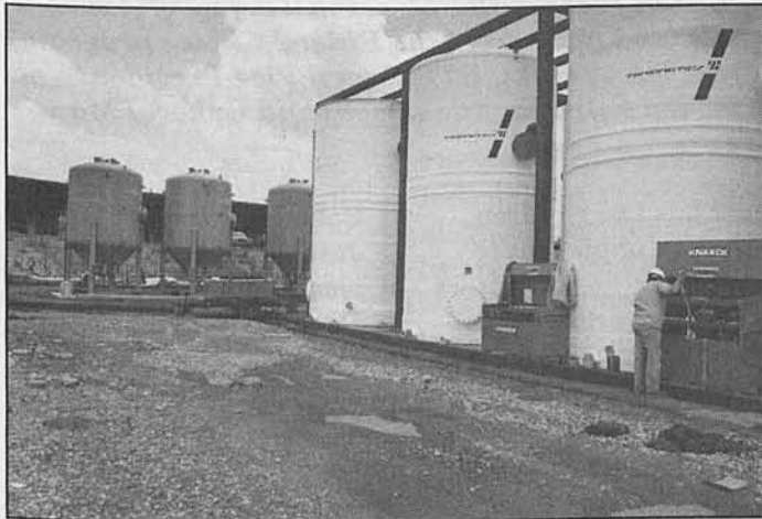
The water treatment plant for Union Station groundwater.
