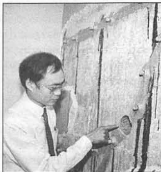
RTD Supervising Engineer Warren Fu inspects repairs of a concrete wall. Core samples were taken to ensure quality control.
