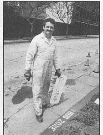
Top left: After sign installing comes painting. Moore swabs the curb with the familiar fire-engine red paint of the bus zone. Stops and Zones uses over 3,500 gallons of red paint a year.
