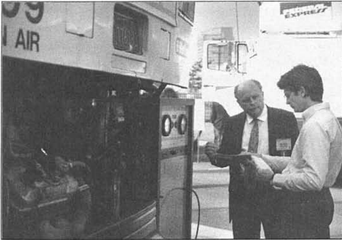
Equipment Maintenance Director Rich Davis informs a reporter about the RTD's refrigerant reclaiming system.
