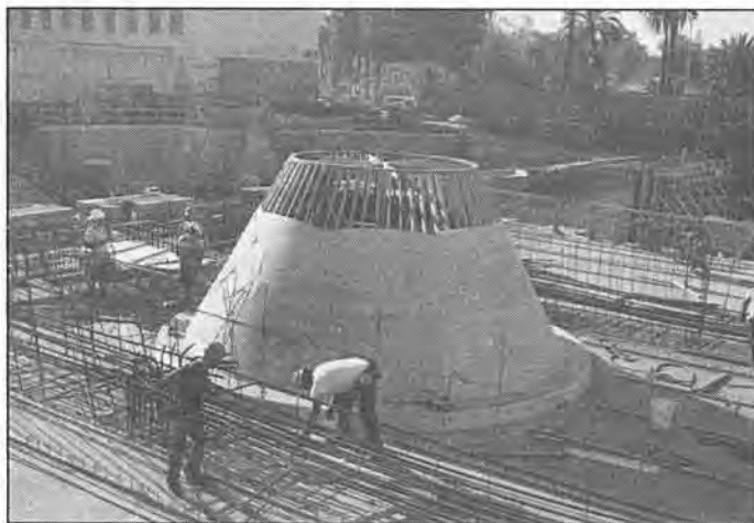
Much further west, workers form the skylight for the Westlake/MacArthur Park station.
