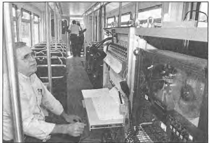
A technician from LTK, an engineering and design consulting firm, at work debugging the electrical system.
