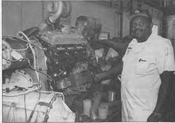
Mechanic A James Evans at work installing the engine oil cooler at Station 8.
