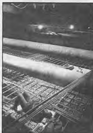
A lady Metro Rail laborer takes her siesta atop the lattice work of rebars at the 4th and Hill Street Station.
