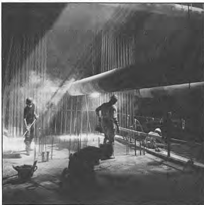
Laborers smooth the foundation of the 7th and Flower Street Station at midday.
