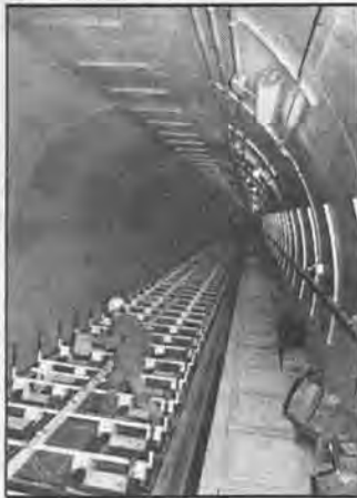
In the Westlake/MacArthur Park tunnel, a mason adds his touch to the pre-track work.
