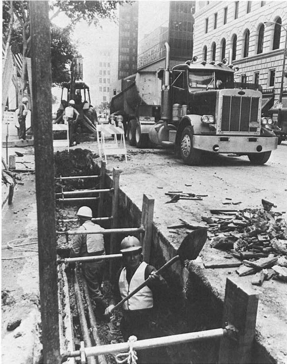
Getting Started —Work crews begin utility relocation work on north side of Seventh Street between Hope and Figueroa as a prelude to tunneling and station excavation.
