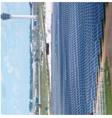
On-site solar array at Indianapolis International Airport Source: www.alleneng.com
