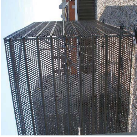
Rooftop HVAC equipment screens with Zero Roof Penetration. Source: www.plaintub.com/
