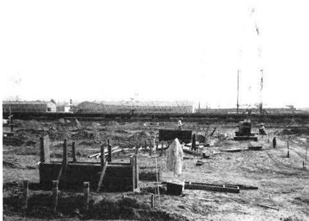
TRACTION POWER STUBUPS, EAST OF MOW BLDG.
