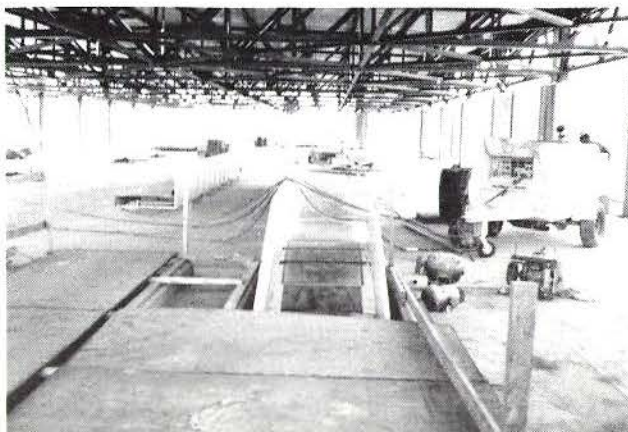
CONVEYOR INSTALLATION AT TRACK LEVEL IN THE BAGGAGE HANDLING FACILITY
