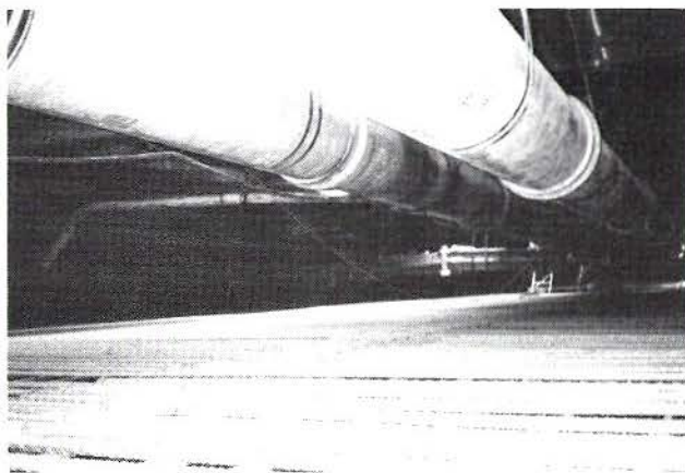
SUPPORTED UTILITIES ABOVE LRT ROOF SLAB
