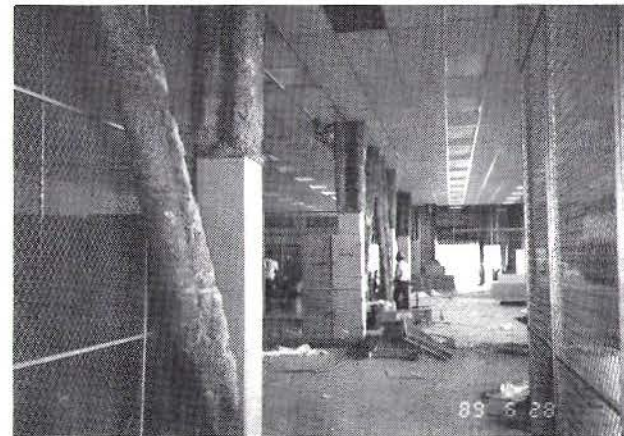
TOOL ROOM & SECURITY STORAGE LEADING INTO SYSTEM STORES
