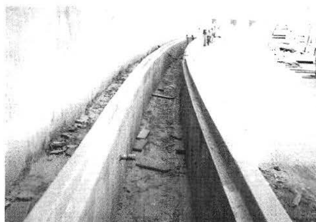
WALKWAY - CABLE TRENCH IN "U" WALL STRUCTURE
