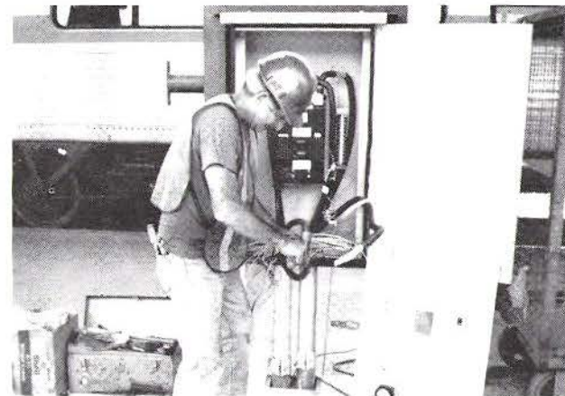
TERMINATION OF ELECTRICAL CABLE AT PLATFORM LIGHTING PANEL
