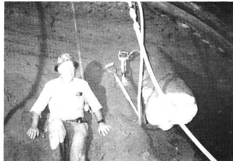
CONCRETE OBSTRUCTIONS (TIEBACKS) ENCOUNTERED DURING EXCAVATION OF CROSS PASSAGE #9
