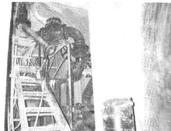
WET STAND PIPE SUPPLY LINE IN CROSSPASSAGE 12
