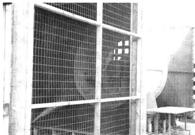
PARALLEL RUN-IN TEST OF EMERGENCY FAN
