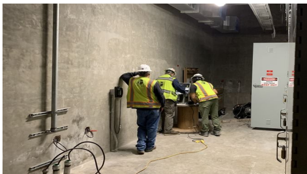
Wilshire/La Brea Station High Potential Testing
