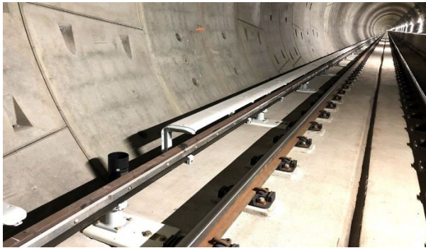
Reach 1 Tunnel Third Rail Cover Board
