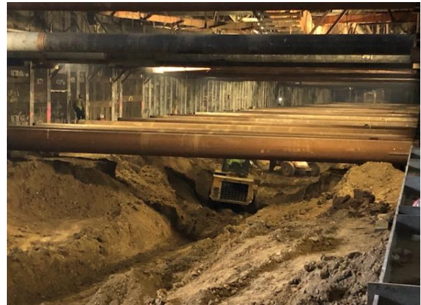
Westwood/UCLA Station: Gut Trench Excavation Under BL2 and BL3 Struts Facing East
