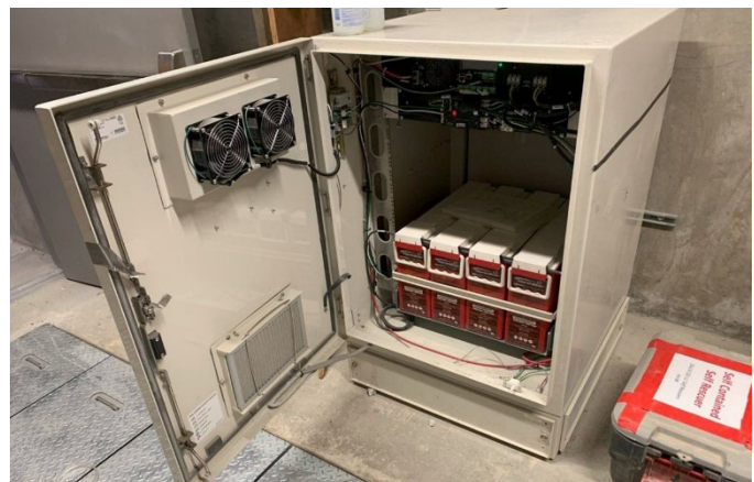
Reach 1 Tunnel (Western to La Brea) UPS System
