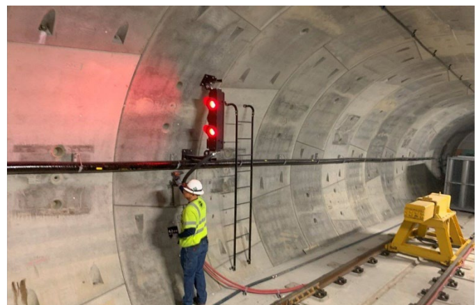
Reach 4 (Tail Track) Tunnel Signal Light Tree
